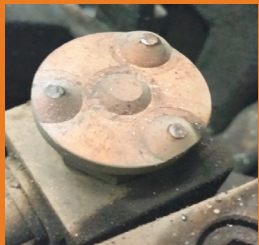
Worn Projection Ground Block
